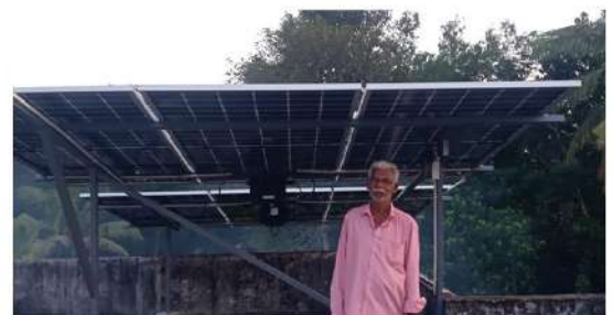
3 kWp On-Grid Solar Power Plant Mr. Mohanan, Kottathala, Kollam
