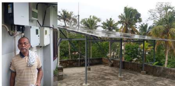
6 kWp On-Grid Solar Power Plant Mr. Ashraf, Oachira, Kollam
