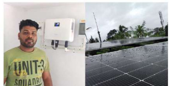
3 kWp On-Grid Solar Power Plant Mr. Junuraj, Paravoor, Kollam
