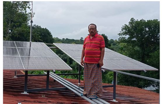
3 kWp On-Grid Solar Power Plant Mr. Jose K George, Chethakkal, Pathanamthitta
