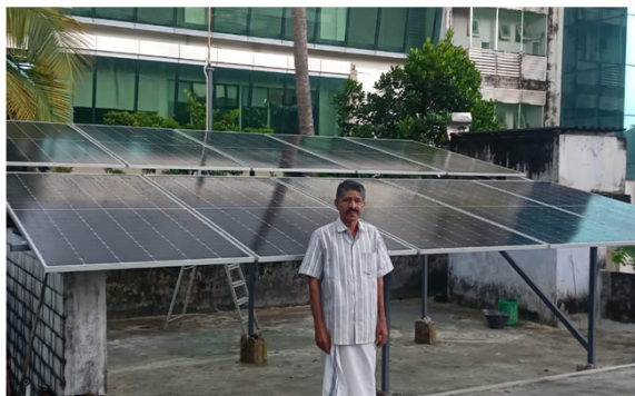
5 kWp On-Grid Solar Power Plant Mr. Kunjachan, Alappuzha
