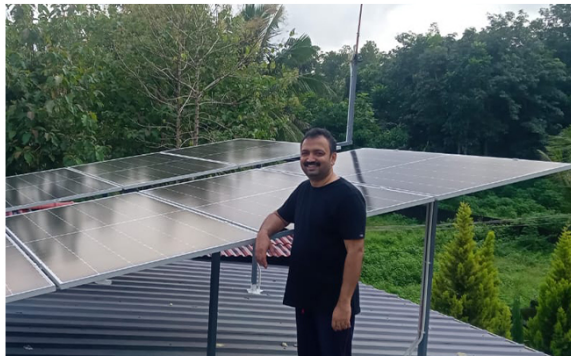
4 kWp On-Grid Solar Power Plant Mr. Josely Abraham, Thiruvalla, Pathanamthitta
