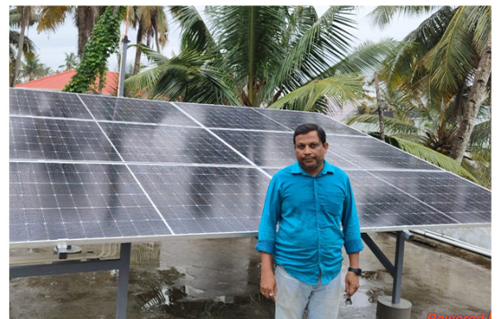
3 kWp On-Grid Solar Power Plant Mr. Bijukumar, Eanchakkal, Trivandrum
