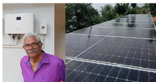
5 kWp On-Grid Solar Power Plant Mr. George, Thrippunitura, Ernakulam
