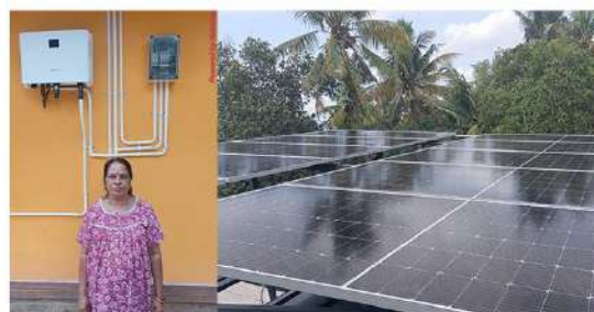
5 kWp On-Grid Solar Power Plant Ms. Jalajakumari, Paravoor, Kollam
