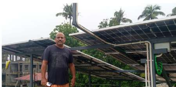
5 kWp On-Grid Solar Power Plant Mr. Shaju, Thrissur
