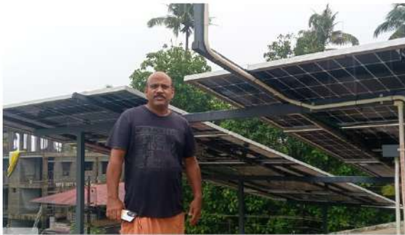
5 kWp On-Grid Solar Power Plant Mr. Shaju, Thrissur
