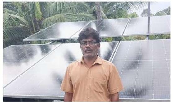
3 kWp On-Grid Solar Power Plant Mr. Satheesh, Kalliyoor, Thiruvananthapuram
