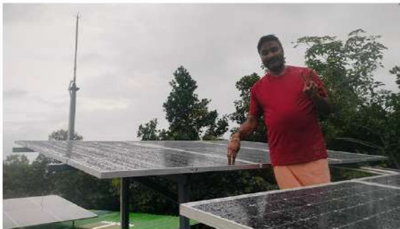
3 kWp On-Grid Solar Power Plant Mr. Santhosh, Mangalapuram, Thiruvananthapuram
