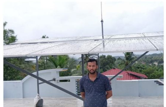
5 kWp On-Grid Solar Power Plant Prashanth K, Nettayam, Thiruvananthapuram
