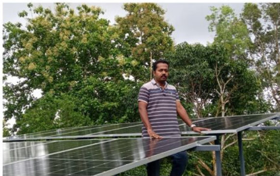
5 kWp On-Grid Solar Power Plant Mr. Mahesh, Sooranad, Kollam
